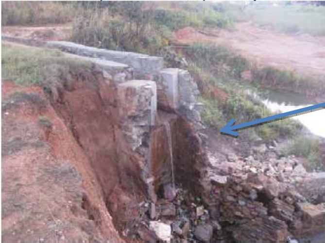
Picture as of 10 April where effluent previously entered the river
