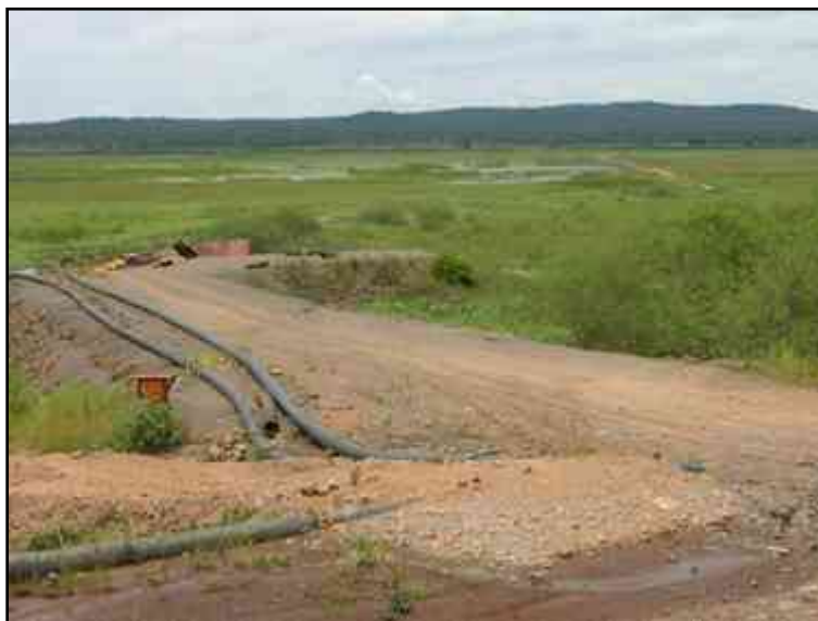
Picture 17: Water pumping station for MUMI plant on the banks of the River Kando (Photo: C.Peyer/BFA)
